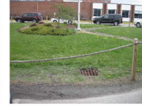
Figure 3: A close-up view of catch basin in the entrance island at front of school that could remain on the overflow from a bio-retention area.
