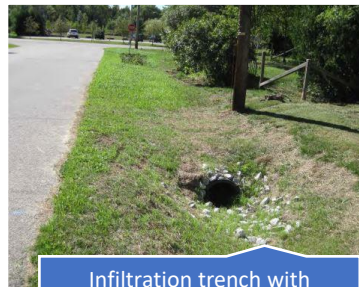
Infiltration trench with perforated pipe to collect runoff
