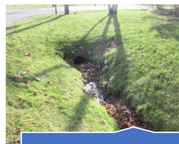
Erosion at the stormwater pipe outlet
