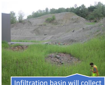
Infiltration basin will collect runoff from gravel pit and garage building
