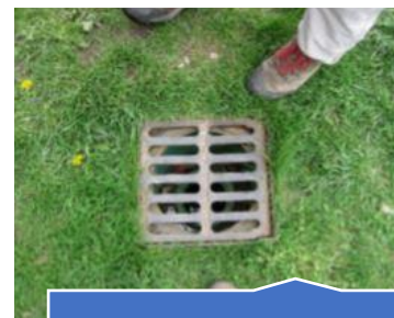
Catchbasin which drains directly to McCabe's Brook, untreated
