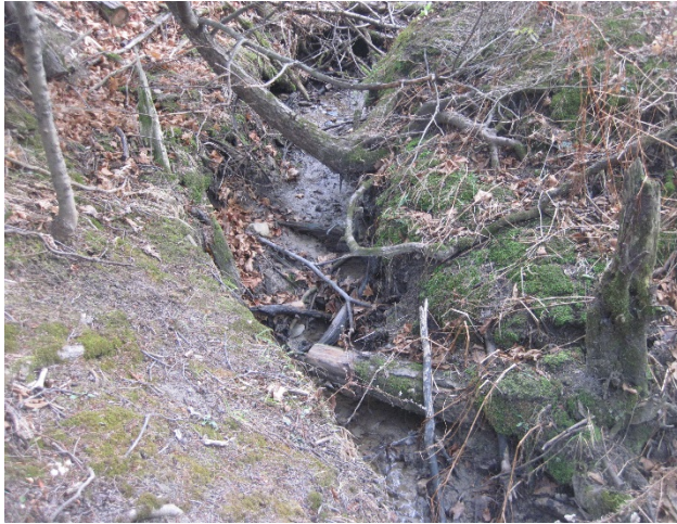
Figure 5: Gully erosion occurring in the channel leaving the neighborhood.
