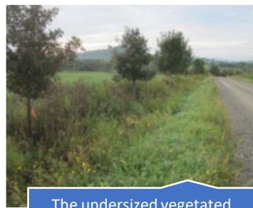
The undersized vegetated swale along E. Thompson's Point Road
