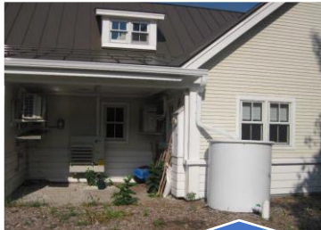
Gutter, downspout, and installed rain barrel for garden watering
