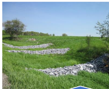
Check dams along a roadside swale slow down water before it reaches Thorp Brook
