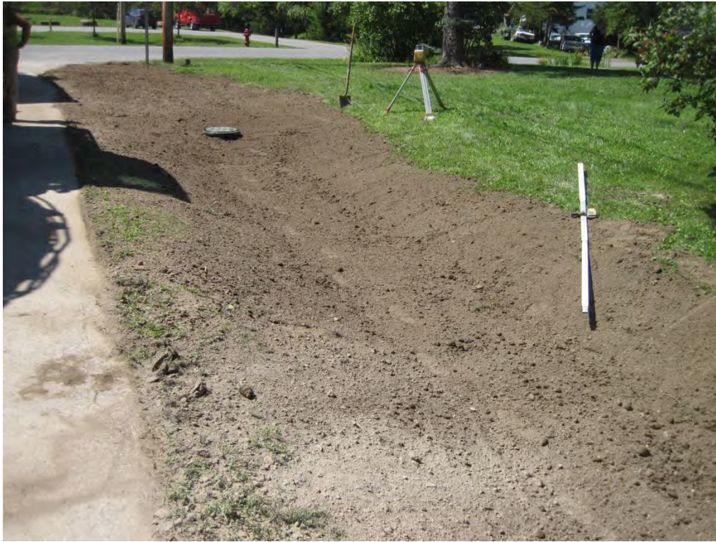
Raingarden area has had topsoil application and fine grading. Waiting on plantings.
