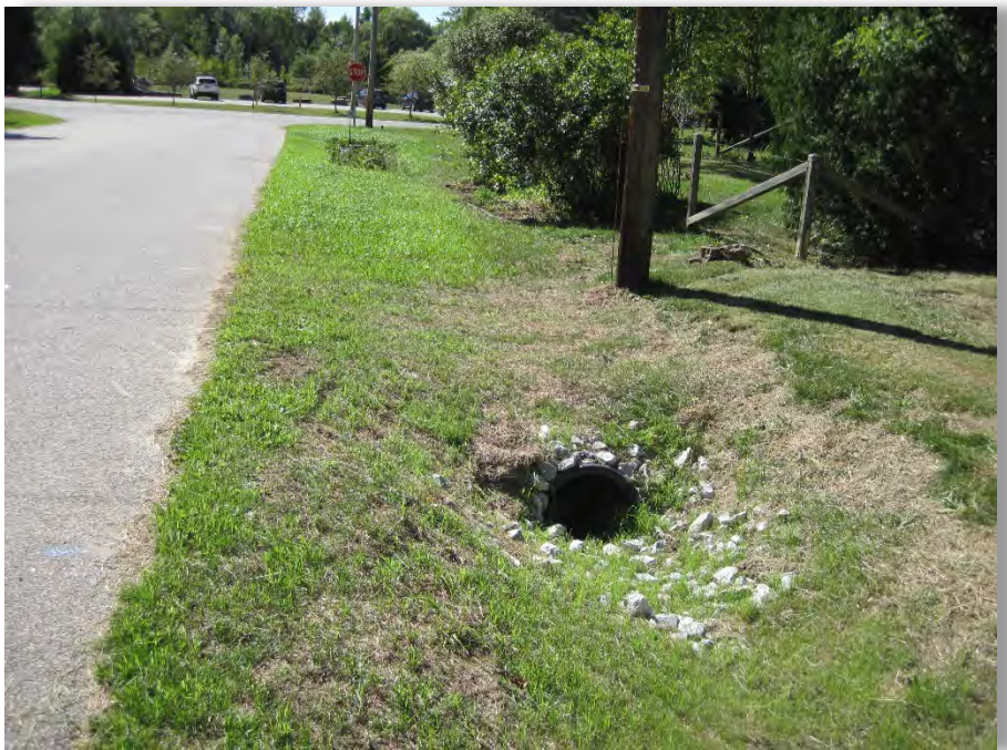
Post-Construction, September 21, 2016: Infiltration trench with perforated pipe installed with shallow grass swale for local surface runoff.
