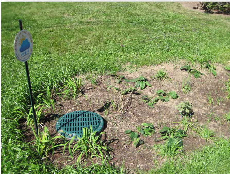
Post-Construction, September 21, 2016: Raingarden created with new flow controlling inlet into downstream infiltration trench.
