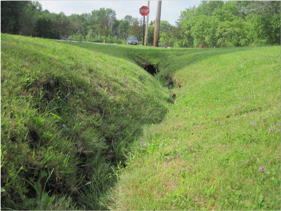
Pre-Construction, July 25, 2016: Steep eroded side slopes of swale do not allow vegetation to grow and create a safety hazard for pedestrians.
