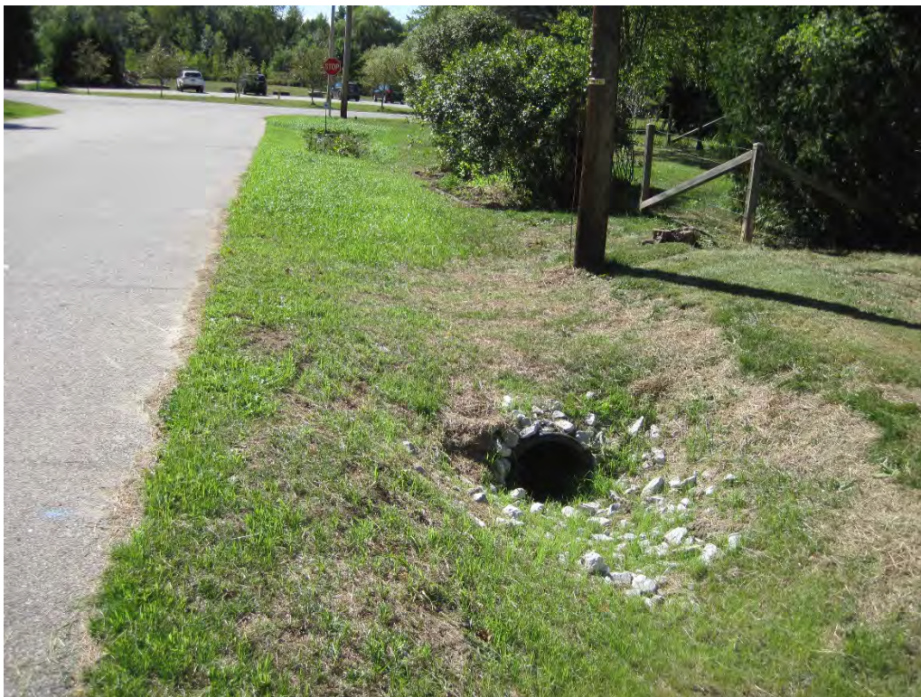
The final grass swale, upstream of the raingarden, viewed looking south along Brook Lane. The infiltration trench and pipe are located below ground. The end of the perforated pipe is visible.
