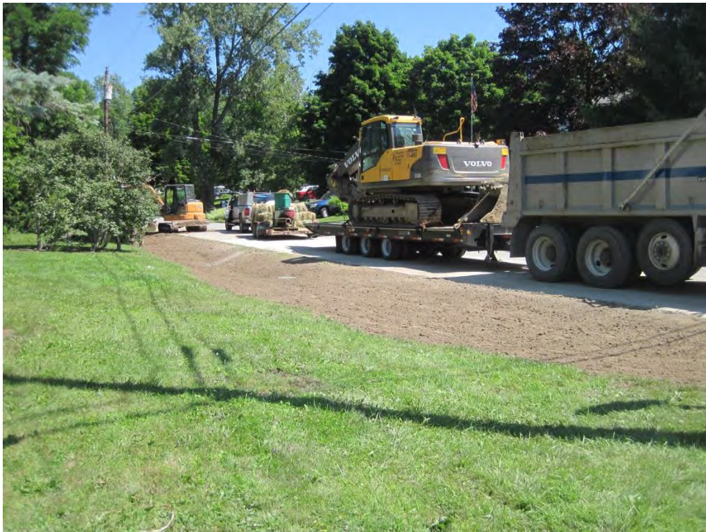
Final grading done over all but last 10 feet, seed applied, mulch application beginning, and equipment loading out.
