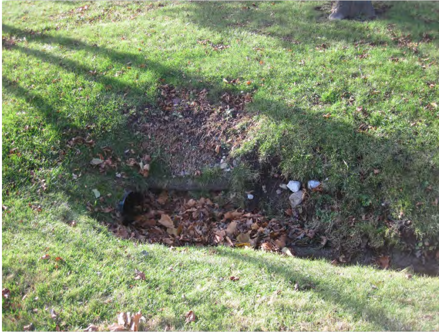
Pre-Construction, November 16, 2012: Erosion at pipe inlet.
