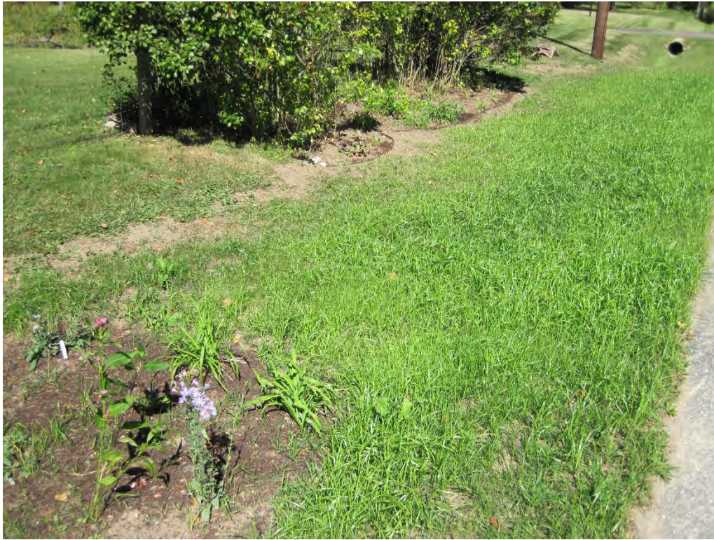
The final grass swale, upstream of the raingarden, viewed looking north along Brook Lane. The infiltration trench and pipe are located below ground.
