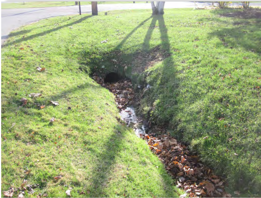
Pre-Construction, November 16, 2012: Erosion and at pipe inlet.
