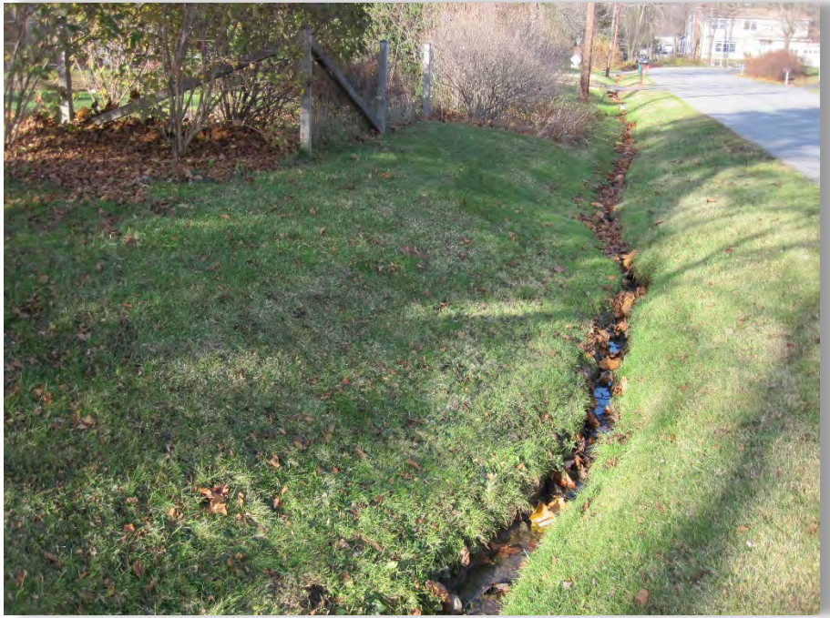
Pre-Construction, November 16, 2012: Erosion along deep narrow swale.
