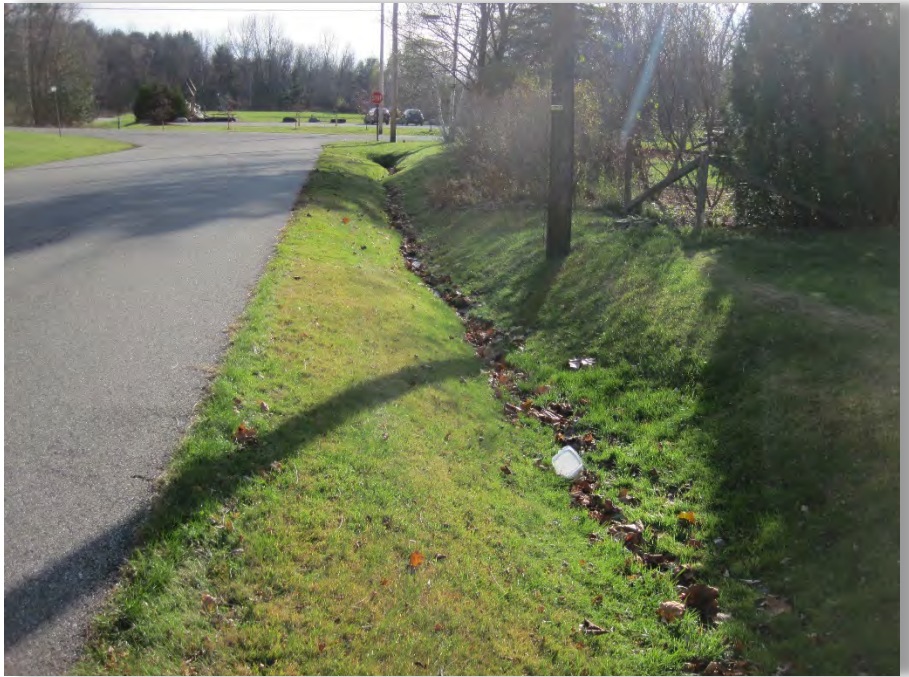
Pre-Construction, November 16, 2012: Erosion along deep narrow swale.
