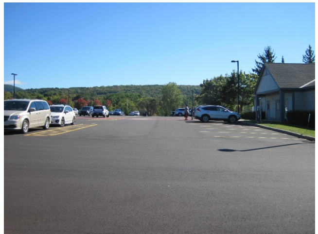
Figure 4: Southwest portion of parking lot and annex building drains to eroding swale at southwest corner of parking area (Recommendation 2).
