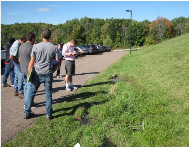
Figure 6: Erosion, puddling, and rutting occurring at the toe of slope between the athletic field/track and north parking lot. This area receives water from underdrains, sheet flow from the parking lot, and a swale draining some of the upper playing fields (Recommendation 1).
