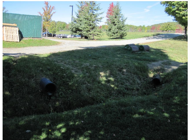
Figure 12: Erosion is occurring in the steep swale and at the entrance and exit of a maintenance driveway crossing. Swale and culvert improvements could slow water and reduce erosion (Recommendation 3).
