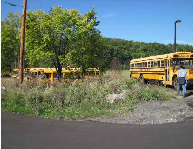
Figure 5: Eroding swale and sparsely vegetated area at southwest corner of parking area could be improved to create bio-retention area and pre-treatment for the fire pond. A catch basin exists in this area, but the grate is set too high to function properly (Recommendation 2).
