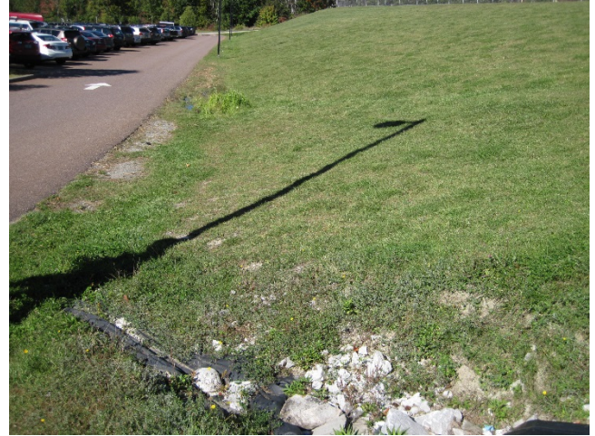
Figure 7: The discharge from the swale at the upper playing fields has some erosion. Swale improvements could help improve water quality as a pre-treatment for the receiving wetland, eventually draining to the fire pond (Recommendation 1).
