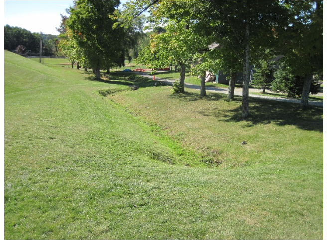
Figure 11: Swales carrying water from the upper playing fields discharges at the east side of the northern parking lot into a steep, eroding swale. This could be a site for a bio-retention area to slow the water (Recommendation 3).
