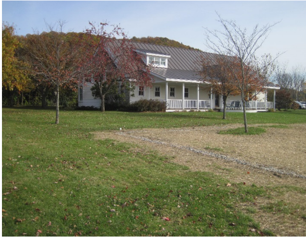
Figure 1: Library existing building, looking across Green. Newly installed gravel perimeter trench drain visible.
