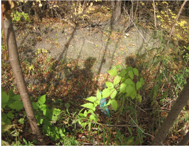
Figure 5: Swale at the north side of the property with some erosion visible.
