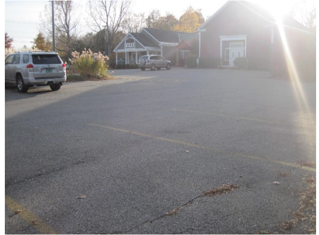
Figure 3: Parking lot draining to catch basins at the east side of the property.
