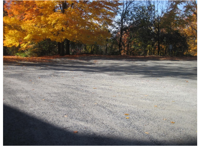
Figure 3: A parking lot to the west of the church has experienced erosion of the gravel surface during rain events.
