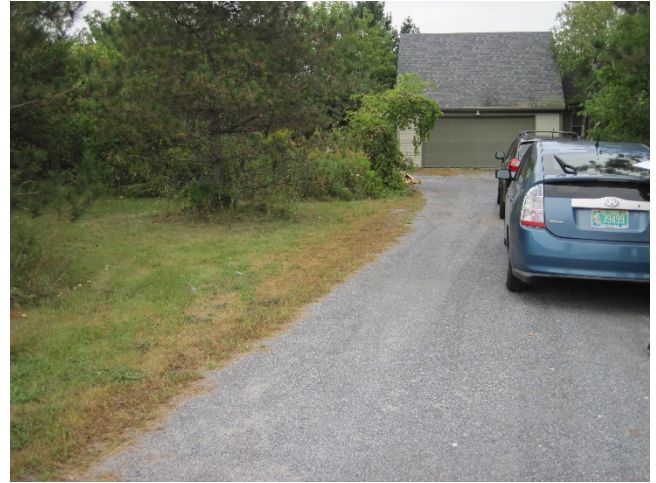
Figure 3: The driveway is low and sloped toward the house, so some water flows towards the house and garage.
