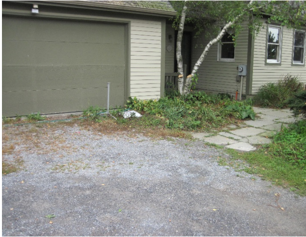
Figure 5: A low spot is located in front of the house and garage.
