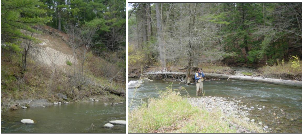
Figure 6.13. Mass Failure in M09A, a source of sediment to the system. Several flood chutes were seen in M09A, signaling planform adjustment.
