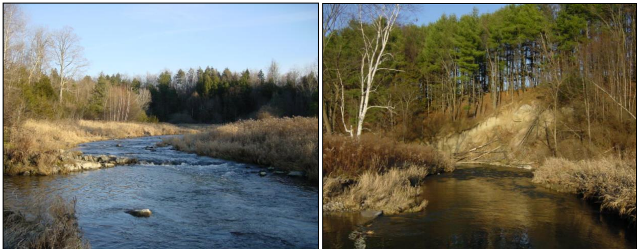
Figure 6.16. Ledge grade control and herbaceous bank vegetation (L), and one of several mass failures in the reach (R).
