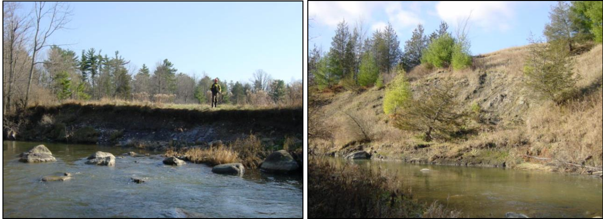
Figure 6.7. Bank erosion on an outside bend, contributing sediment (L) and one of many mass failures in M06 (R).
