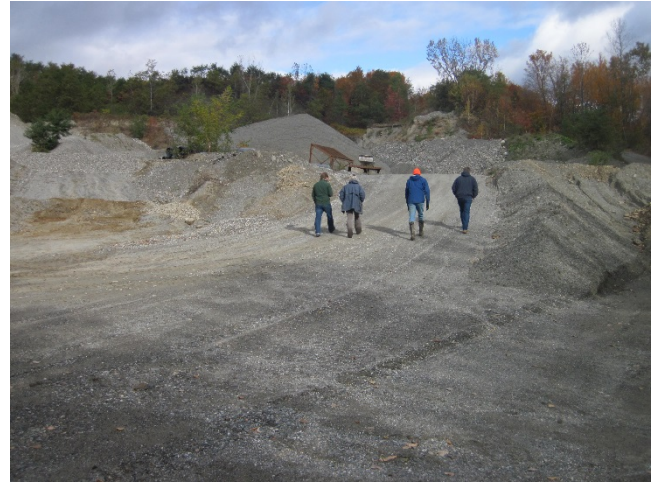
Figure 3: The active gravel pit excavation area is located at a higher elevation than the buildings.
