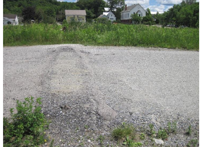
Figure 15: Heaved 18 inch corrugated metal pipe under Stella Road (June 23, 2021).
