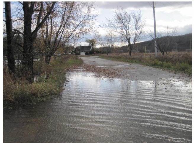
Figure 12: Stella Road partially flooded looking south from junction with drive to Cheese factory gravel parking area (November 1, 2019).
