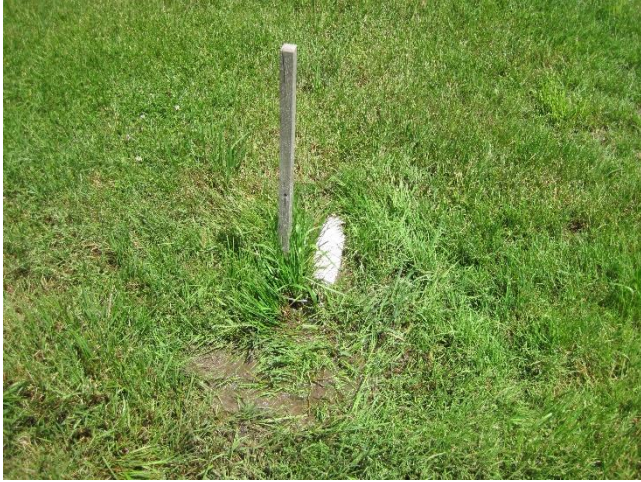
Figure 21: 3 inch PVC drainage pipe extending from church into mowed lawn area (June 23, 2021).
