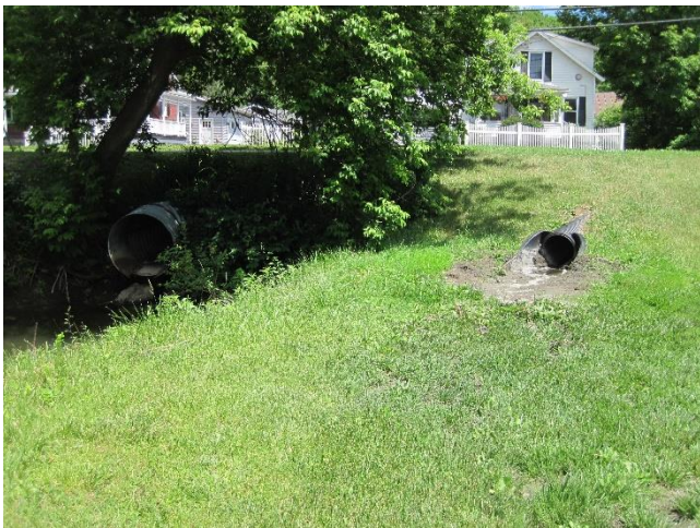
Figure 2: Outlet of 36 inch corrugated metal pipe under Route 116 and 15 inch plastic stormwater culvert (June 23, 2021).
