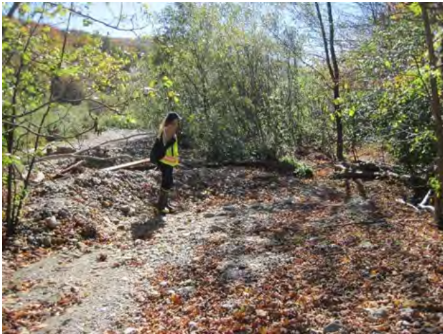
Figure 5: Flows left Hollow Brook in several spots and carried materials into the field, as shown on the left side of this photo (October 9, 2020).
