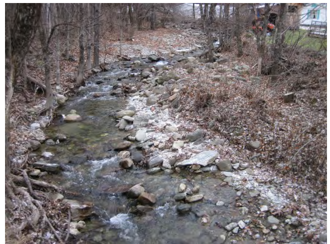
Figure 12: A view of the channel looking upstream from on top of the culverts (December 6, 2020). Large sediment deposits fill the channel, covering tree bases.
