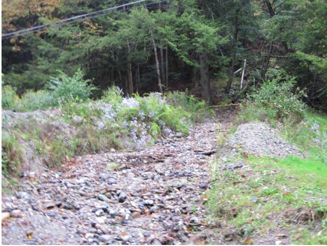
Figure 21: Sediment has washed down into the Hollow Brook channel and has been bermed up on both sides to recreate the path to the river where sediment has deposited (October 2, 2020).
