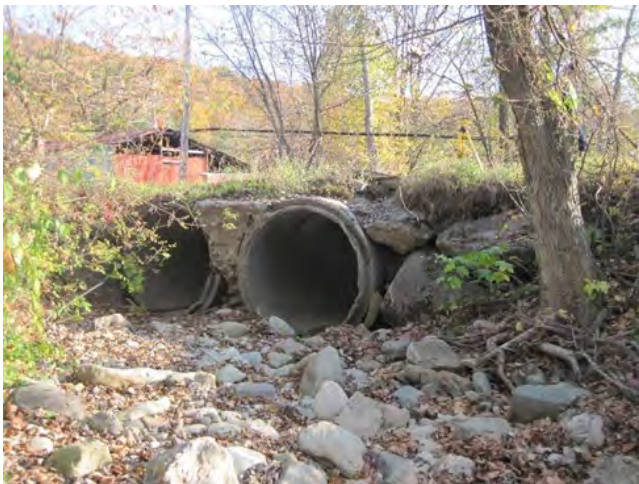
Figure 10: The channel begins to go dry at the culverts (October 9, 2020). A view of the culverts from upstream.
