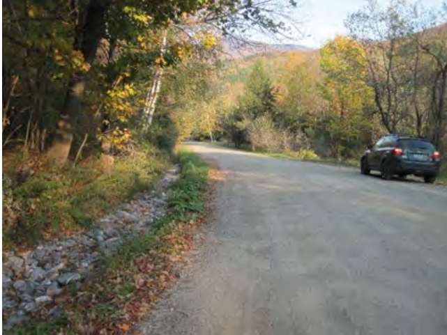
Figure 17: Stormwater from Lincoln Hill Road is collected in road ditches and directed to a Hollow Brook tributary (October 9, 2020).
