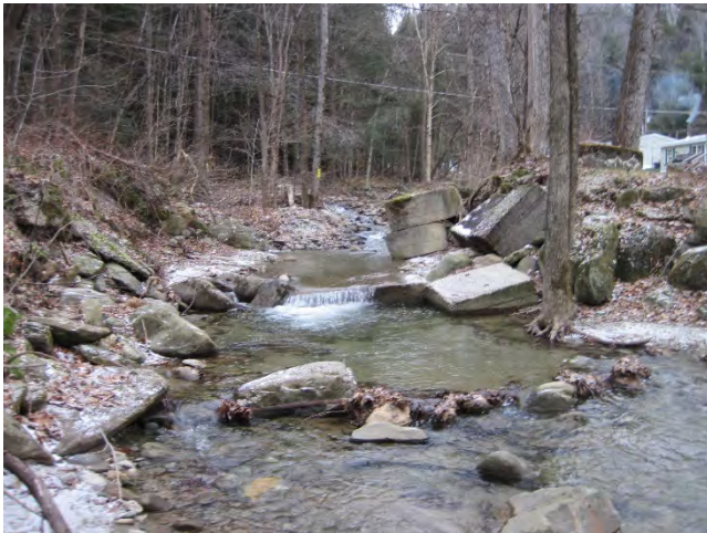
Figure 14: A concrete sill crosses the river at an abandoned crossing. Abutments constrict channel to 12.5' wide. View of old bridge abutments looking upstream (December 6, 2020).
