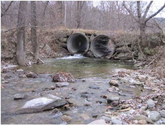
Figure 9: The driveway culverts are perched with a scoured pool at the downstream end of the culverts (December 6, 2020).
