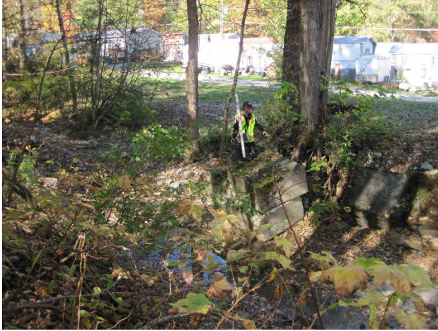
Figure 13: When flow backs up at the old abutment constriction, the water flows out onto nearby Elm Lane, damaging homes, and carrying sediment (October 9, 2020).
