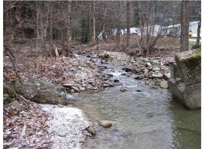
Figure 15: View of old bridge abutments looking upstream. There is a steep riffle and sediment deposit filling the river channel and contributing to flows leaving the channel (December 12, 2020).
