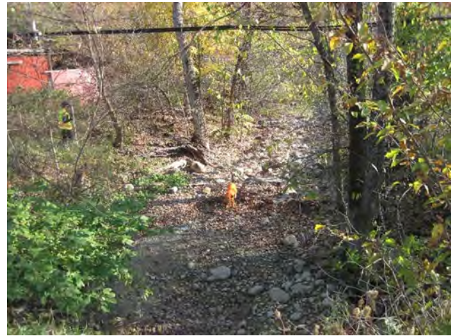
Figure 11: A view of the channel looking downstream from on top of the culverts (October 9, 2020).
