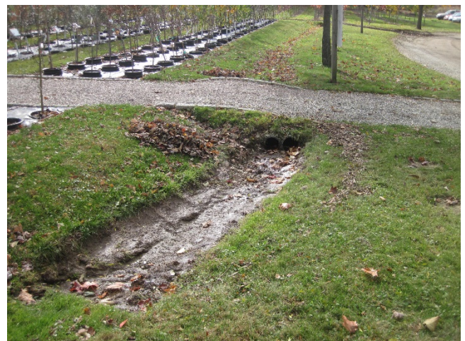
Figure 4: A swale system with small culverts carries water around the site, but requires frequent maintenance.
