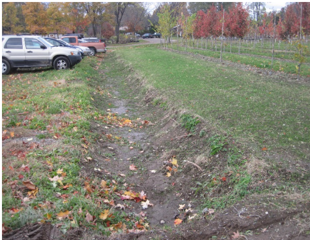
Figure 6: A swale carries water from the entrance area and many of the planted nursery fields to the south off of the site.
