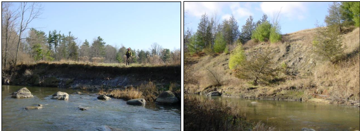
Bank erosion on an outside bend, contributing sediment (L) and one of many mass failures in M06 (R).
