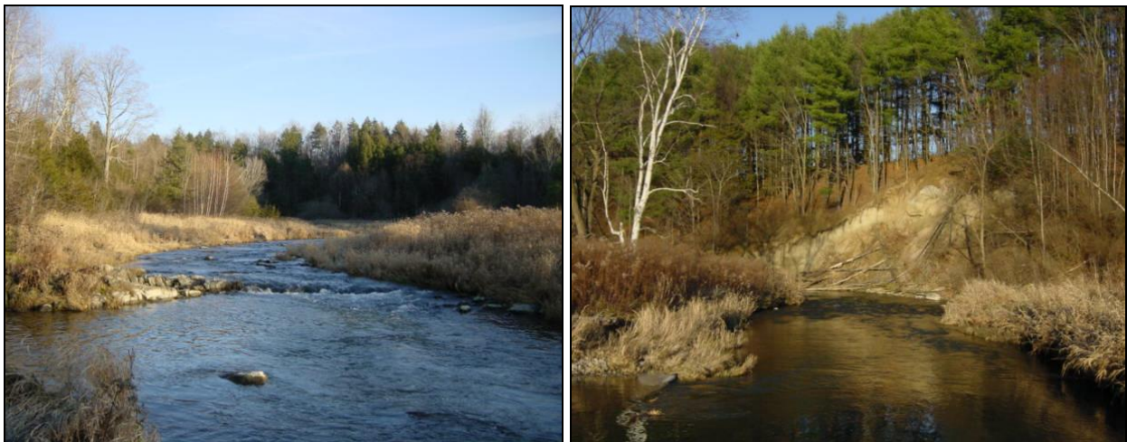
Ledge grade control and herbaceous bank vegetation (L), and one of several mass failures in the reach (R).
