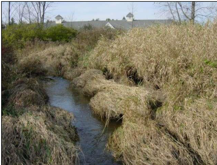
Bank slumping in T1.03.
