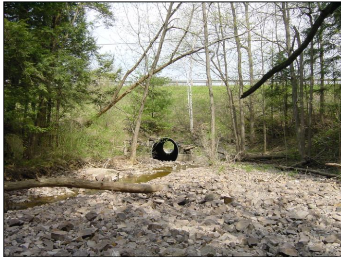
Bostwick Rd crossing in T1.05A with large sediment deposits and channel widening upstream.
