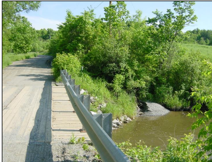
Leavensworth Road and bridge at M12 with large sediment deposit on the right where the road ditch meets the channel.
