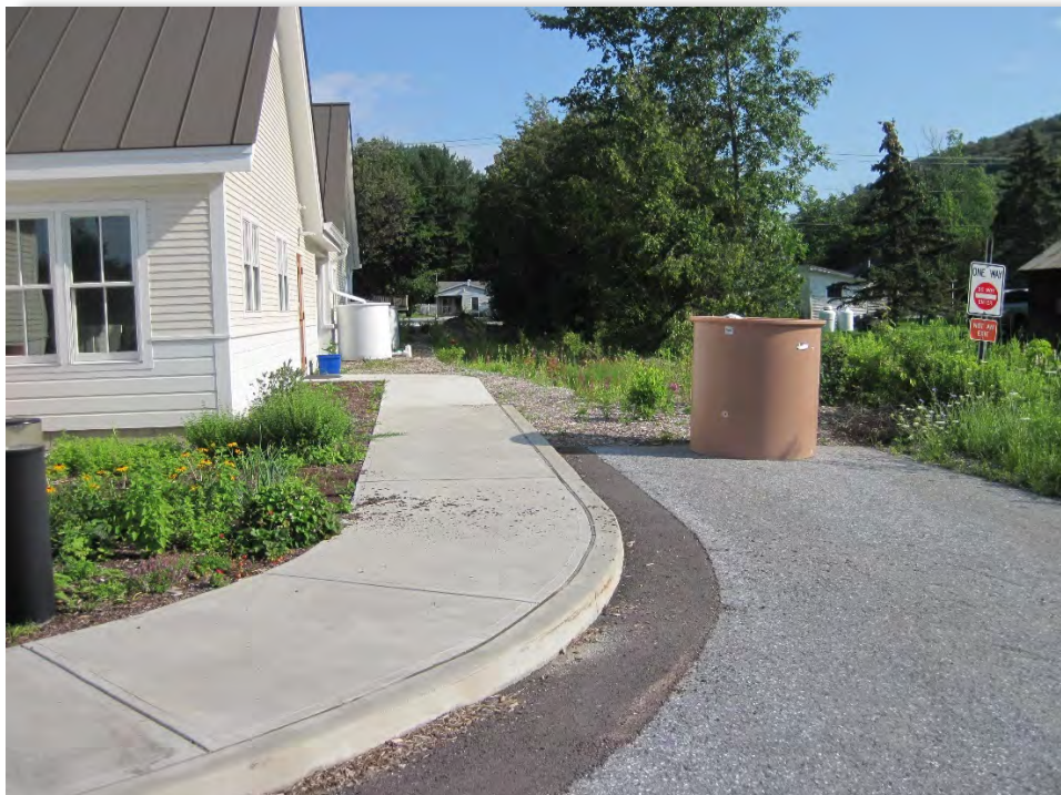
Post-Construction, July 23, 2021: A portion of the impervious surface from the library entrance driveway has been removed and a bio-retention area has been installed fed by overflow from rain barrels collecting roof runoff.
