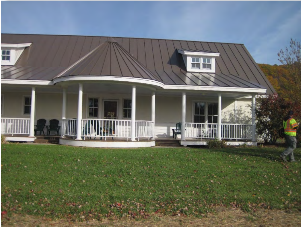
Pre-Construction, October 27, 2015: West side of the library. Roof runoff currently falls off roof and travels overland into the Green.
