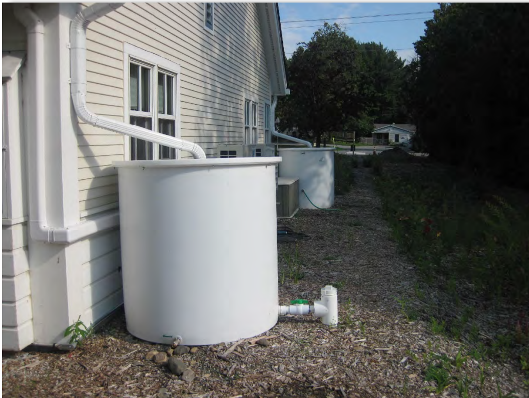
Post-Construction, July 23, 2021: The rain barrels collect runoff from the east side of the building.
