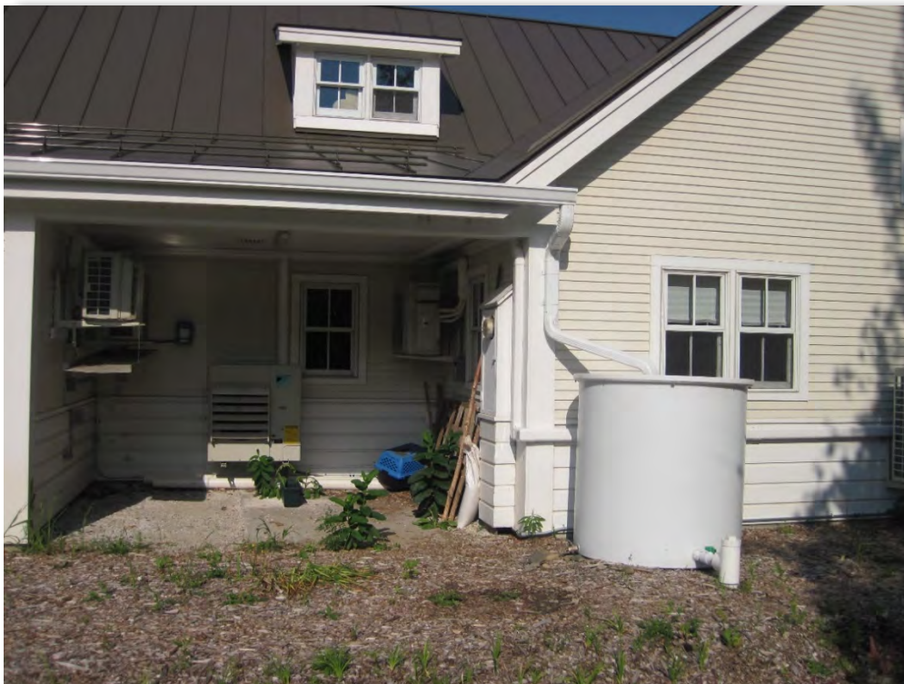
Post-Construction, July 23, 2021: Gutter, downspout, and rain barrel installed. Overflow from this rain barrel flows into the bio-retention area. Runoff collected in the rain barrel will be used for garden watering.
