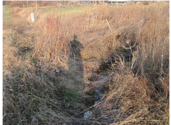
Figure 4: The swale from the north turns sharply to the east, joining the East Thompson Point Road swale.
