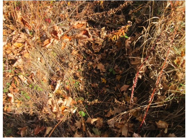
Figure 6: Active erosion in the swale adjacent to the horsepath, partially hidden by vegetation.
