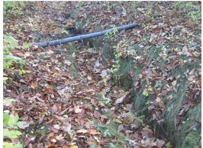
Figure 11: Active gully erosion in the cross-slope swale, partially hidden by vegetation.
