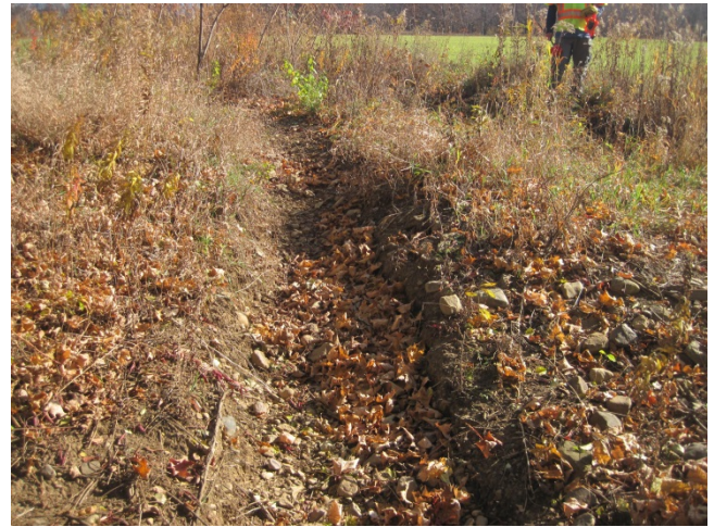
Figure 5: Erosion is actively occurring along the horsepath and in the adjacent swale (hidden in vegetation).
