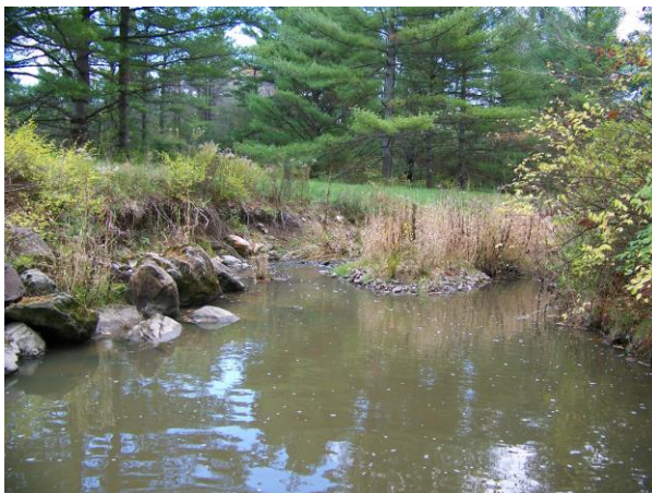
Failing riprap and bank erosion along the pond and possible berm.
