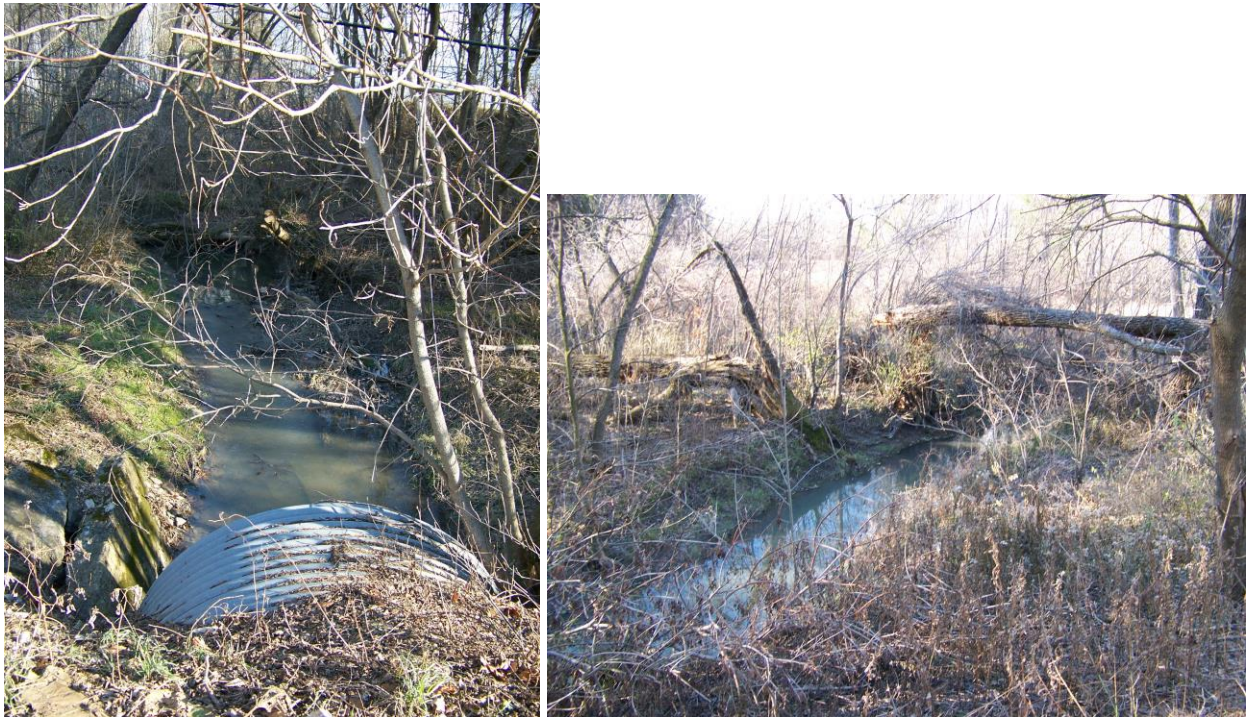
View of a culvert and bank erosion (L) and the stream channel (R).
