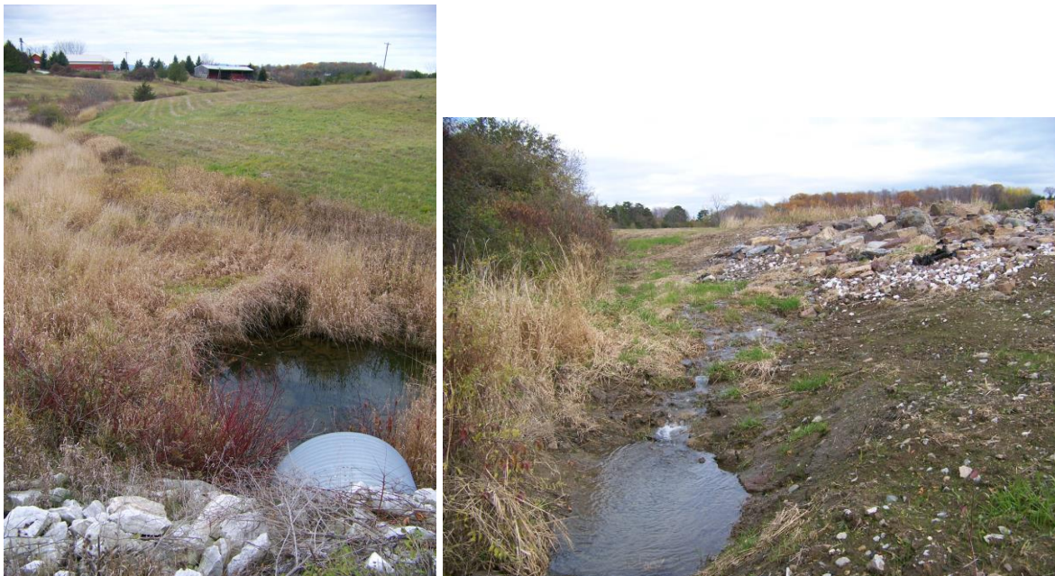
View of culvert, fields and grassy stream banks (L); view of downstream end of pond/dam with recent repairs and flow emerging (R).
