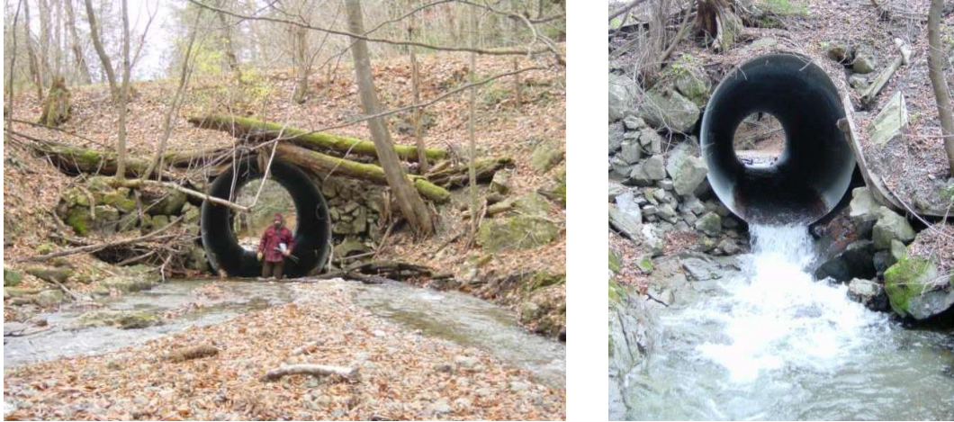
Figure 7. Beecher Hill Brook (T5.01B) culvert. Note aggradation forming bars and splitting flow upstream. Some erosion was noted downstream, although the downstream end falls onto ledge and boulders.
