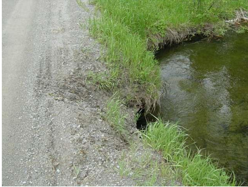
Figure 9. Sand and gravel from roads washing into the channel.
