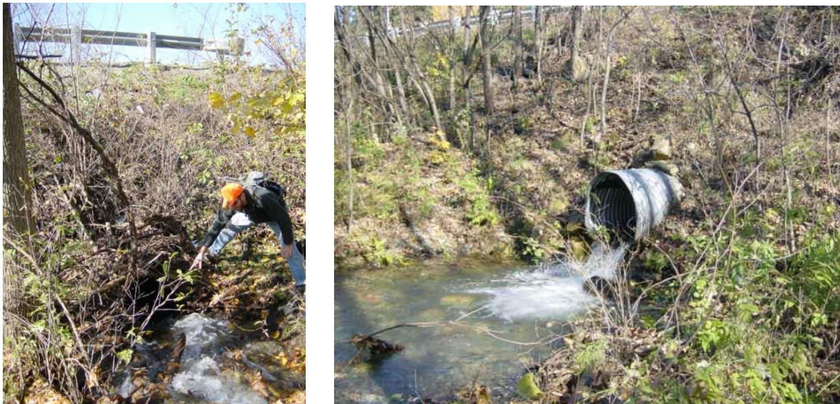
Figure 8a. Culvert on segment M18B. The upstream end of the culvert was blocked by sediment and debris and was hardly visible (left). Extreme scour was apparent at the downstream end and beyond (right).
