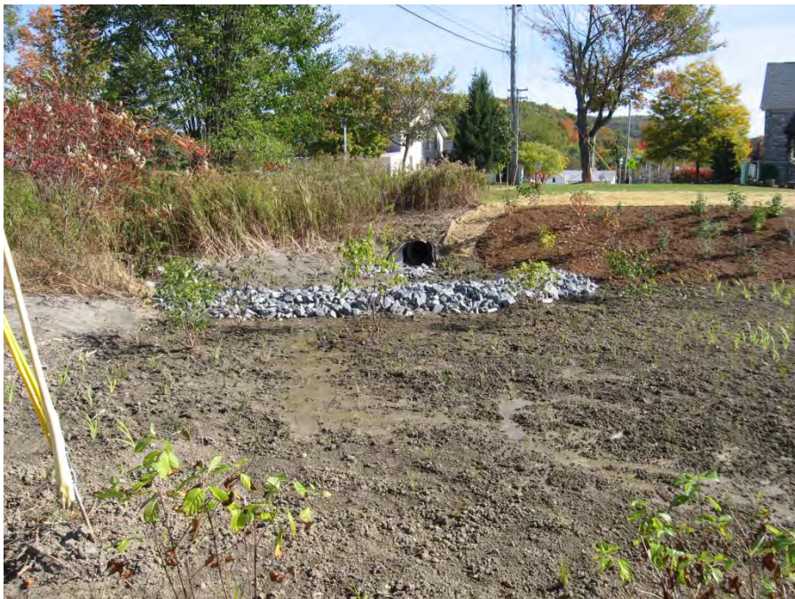
Post-Construction, October 3, 2014: View of completed upper treatment cell and sediment forebay looking east.
