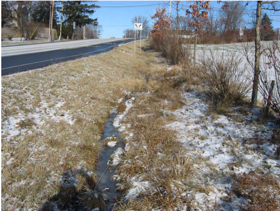
Pre-Construction, December 12, 2012: View of existing eroding swale along Silver Street looking north.
