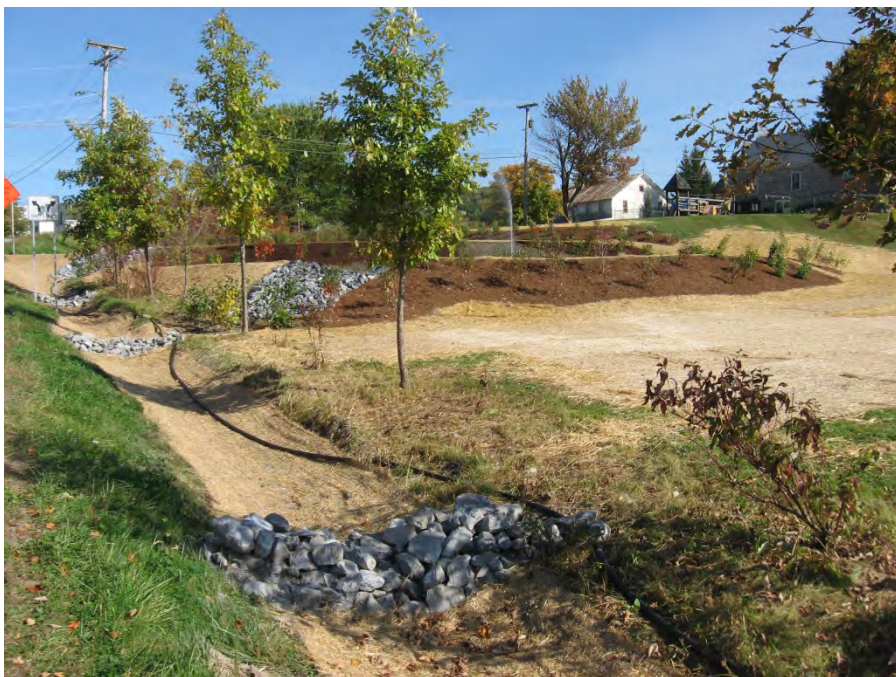
Post-Construction, October 3, 2014: View of completed swale and lower treatment cell looking north.
