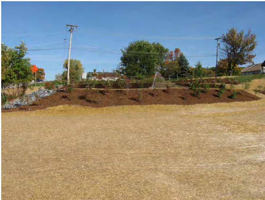
Figure 5: View of completed rain garden treatment cells from the school parking lot / site access point. Erosion control matting used to recover the site visible in the foreground.
