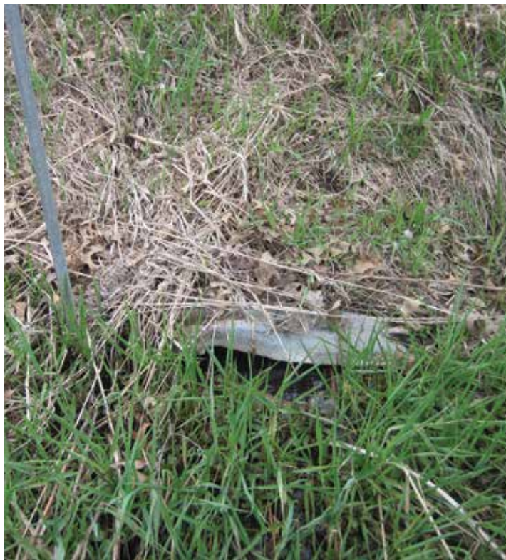
Problem: culvert crushed and blocked
