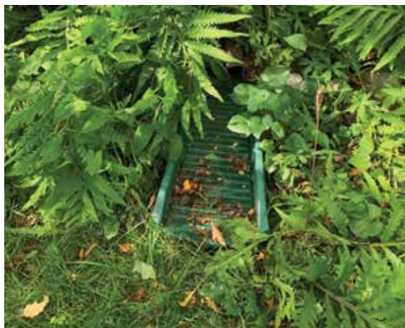
Downspout level spreaders take water from gutter downspouts and spread it out into the lawn to avoid erosion.
