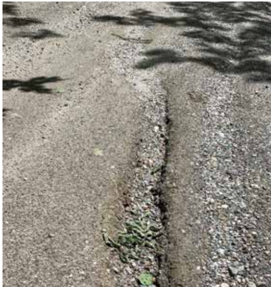
Problem: driveway erosion in wheel ruts
