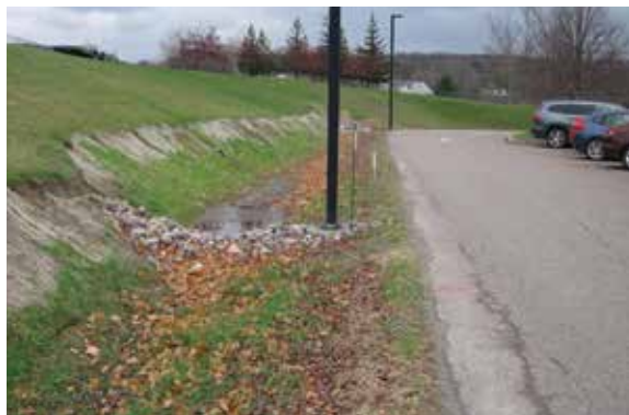
Check dams slow down and hold back water as it travels down a swale.
