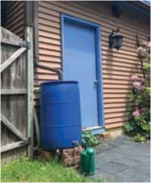
Downspout directed into rain barrel
