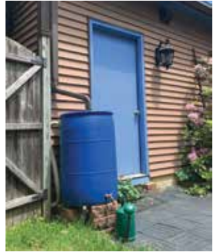
Downspout directed into rain barrel
