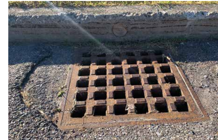
Problem: stormwater and pollutants, like sediment, drain to the Winooski River, with no treatment
