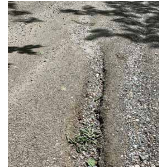
Problem: driveway erosion in wheel ruts
