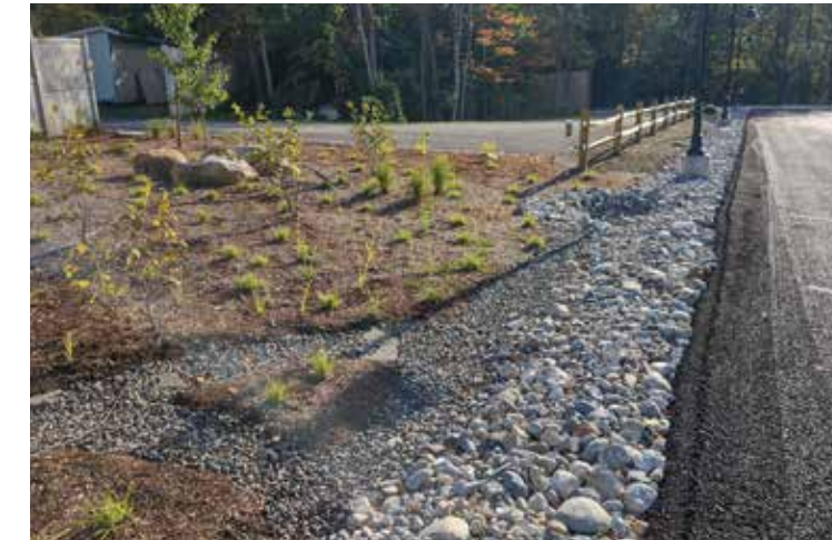
Infiltration trenches allow water to flow into stones and seep into surrounding ground.
