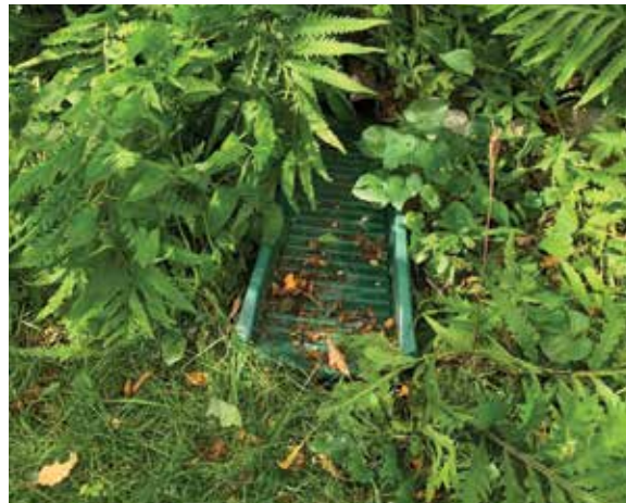
Downspout level spreaders take water from gutter downspouts and spread it out into the lawn to avoid erosion.
