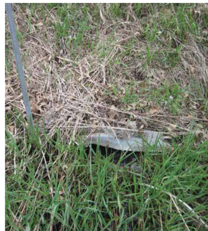
Problem: culvert crushed and blocked
