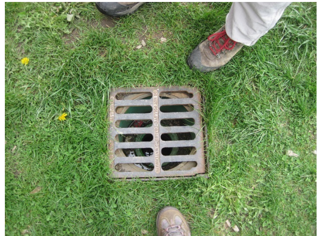
Figure 12: A grate inlet, typical of the series that runs around the south and west sides of the school.
