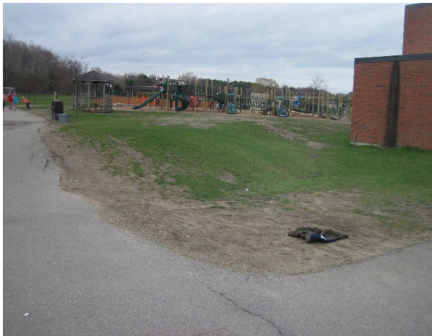
Figure 10: The lawn and dirt area where the roof runoff travels across is a high-traffic area leading to the playground.
