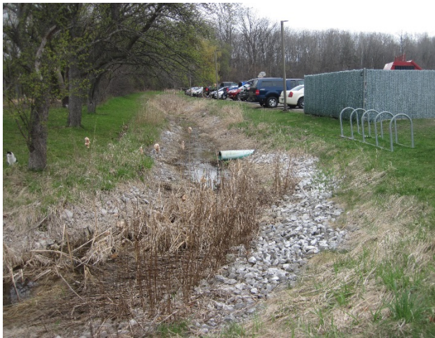
Figure 6: To the north of the tennis court the swale carrying water from the upper part of the subwatershed is in a uniform rock lined swale with minor vegetation and no buffer from the parking lots or dumpsters.
