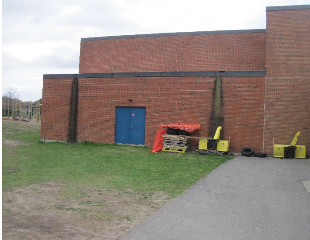
Figure 9: Roof runoff runs down the side of the roof at two locations off of the storage area adjacent to the gyms. It is staining the brick and runs across lawn to a catchbasin.
